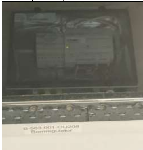
Bilde 02, Romregulator montert over himling
